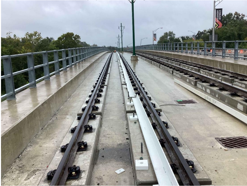
S28 Anacostia LRT Bridge over NE Branch - Site View of the direct fixation track #1 and #2 and overhead catenary system work progress (09.10.25)
