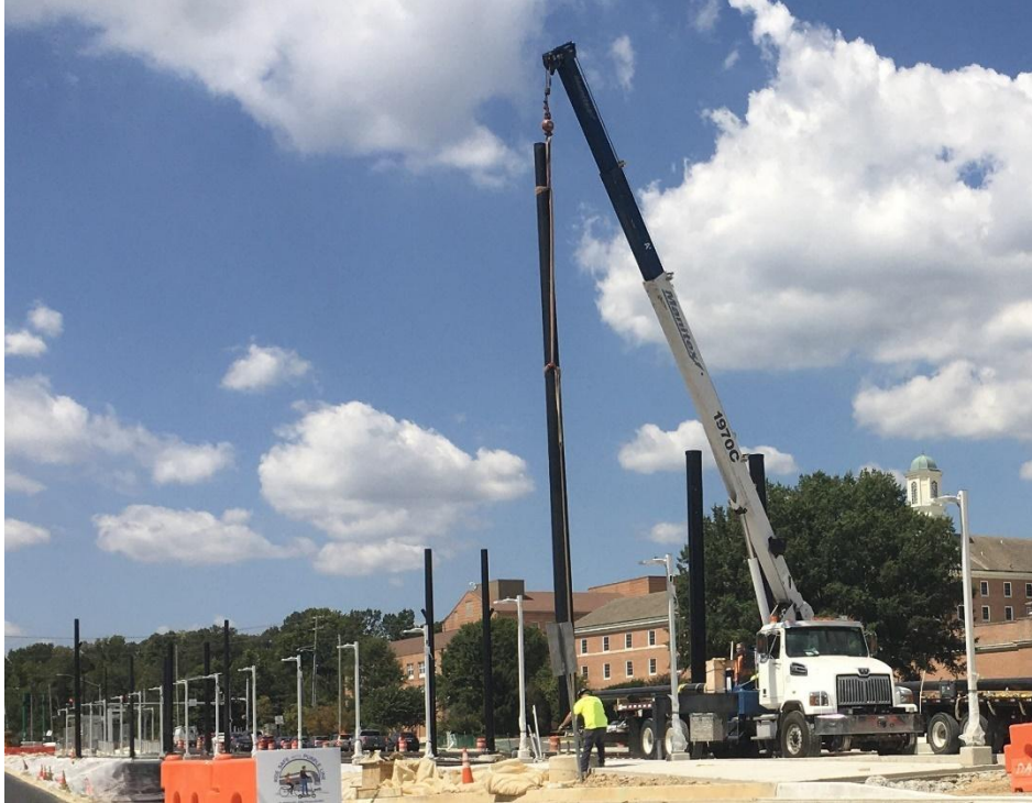
Site View of overhead catenary system poles installation work progress on Campus Dr at Adelphi Road-UMGC-UMD Station. (09.03.25)
