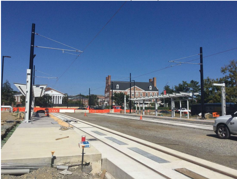
Site view of the overhead catenary system messenger wiring work along Rossborough Ln at the Baltimore Ave.-UMD Station. (09.05.25)
