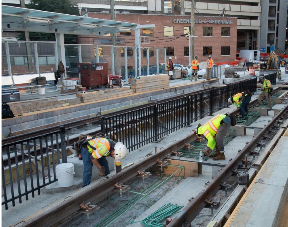
Direct Fixation Track - Site view of track #1 and #2 work progress at Silver Spring Station (09.04.25)
