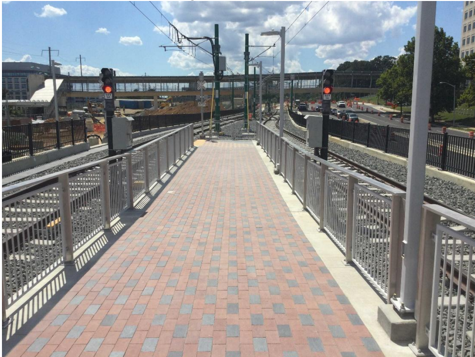
New Carrollton Station - Site View of the platform art in transit pavers and track signal installation work progress along Ellin Road. (08.28.25)
