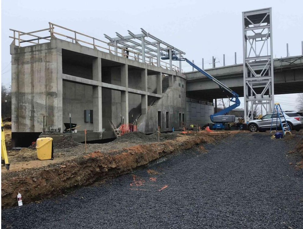
Segment 2 (Lyttonsville Yard area): Lyttonsville Station – Site view of the Station canopy and elevator work progress. (12.10.24)
