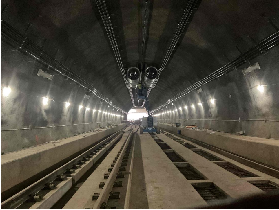
Segment 4 (Manchester Road to Arliss Street / Plymouth Tunnel): Plymouth Tunnel – Site view of jet fan installation work progress. (01.24.25)
