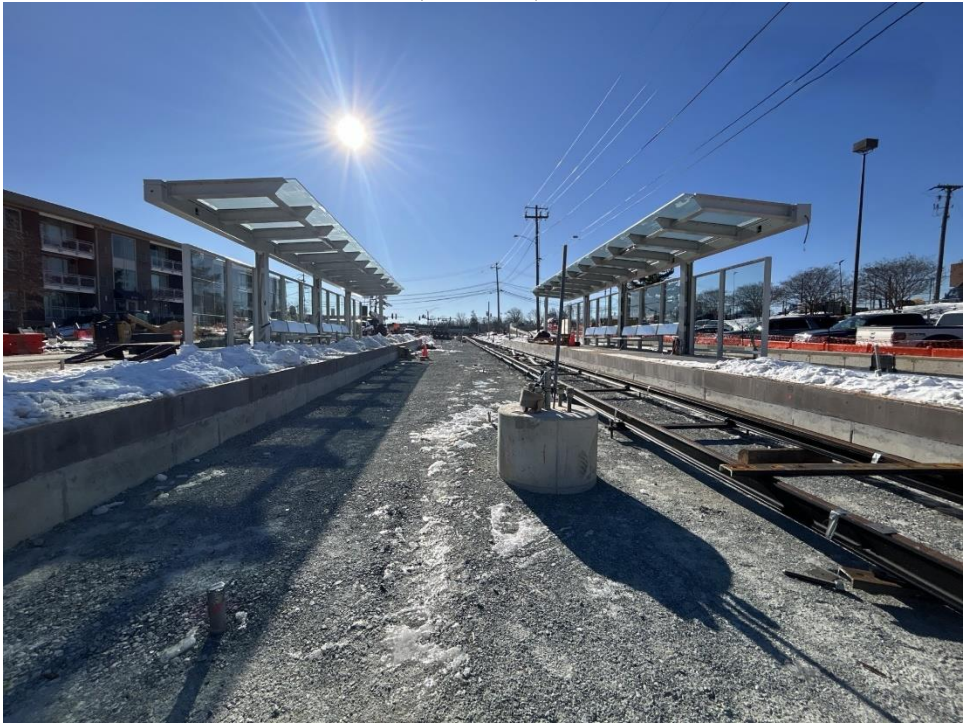
Long Branch Station – Site view of platform canopy and windscreen frame work progress. (01.15.25)
