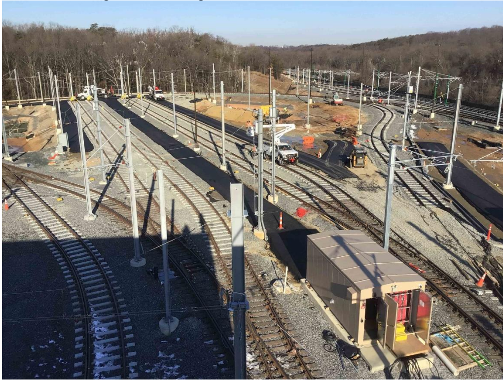
Site View of Glenridge Yard looking East at the ballast track and OCS work. (01.31.25)
