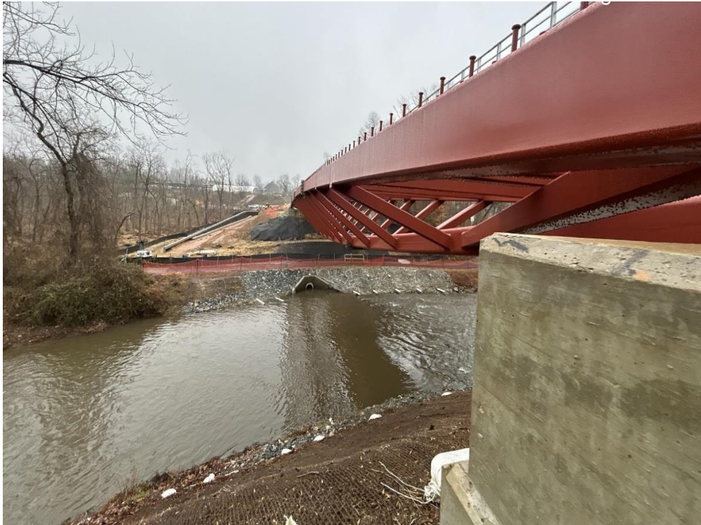
Rock Creek Capital Crescent Trail (CCT) Bridge - Site view of the S14 CCT pedestrian bridge structure set in place over Rock Creek. (12.16.24)
