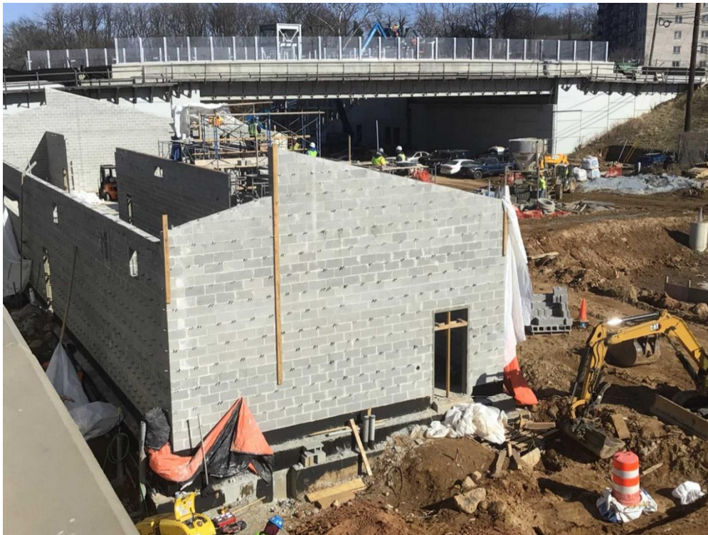
Lyttonsville OMF - Site view of the concrete masonry unit work for the walls. (01.28.25)
