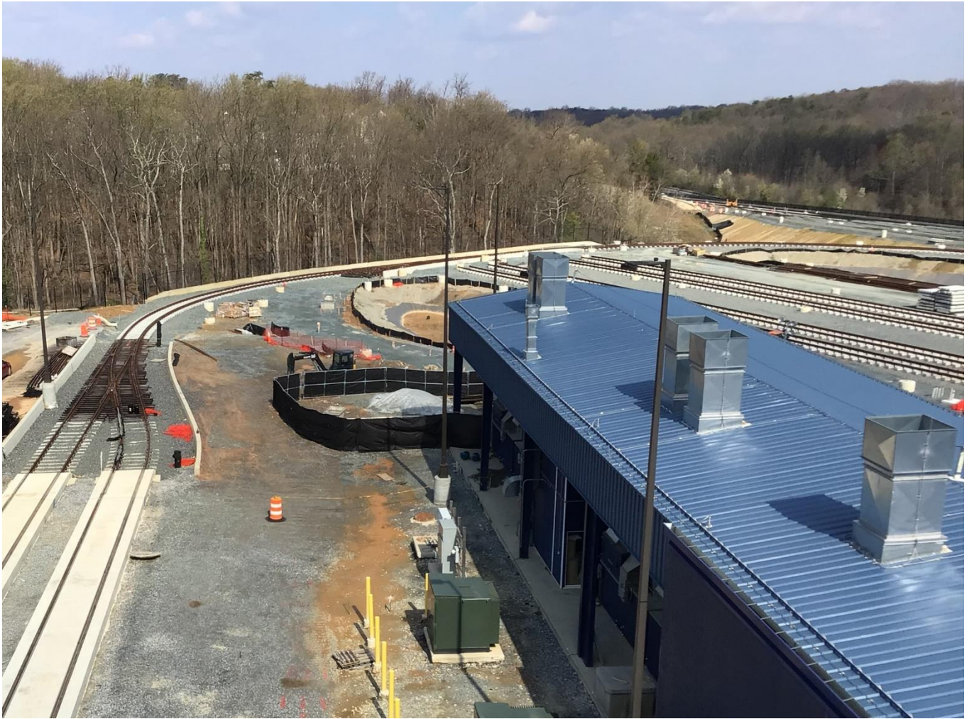
Segment 8: Embedded track connection to ballast MOW tracks around the paint booth inside the Glenridge Yard Facility heading towards MD450. (03.29.24)
