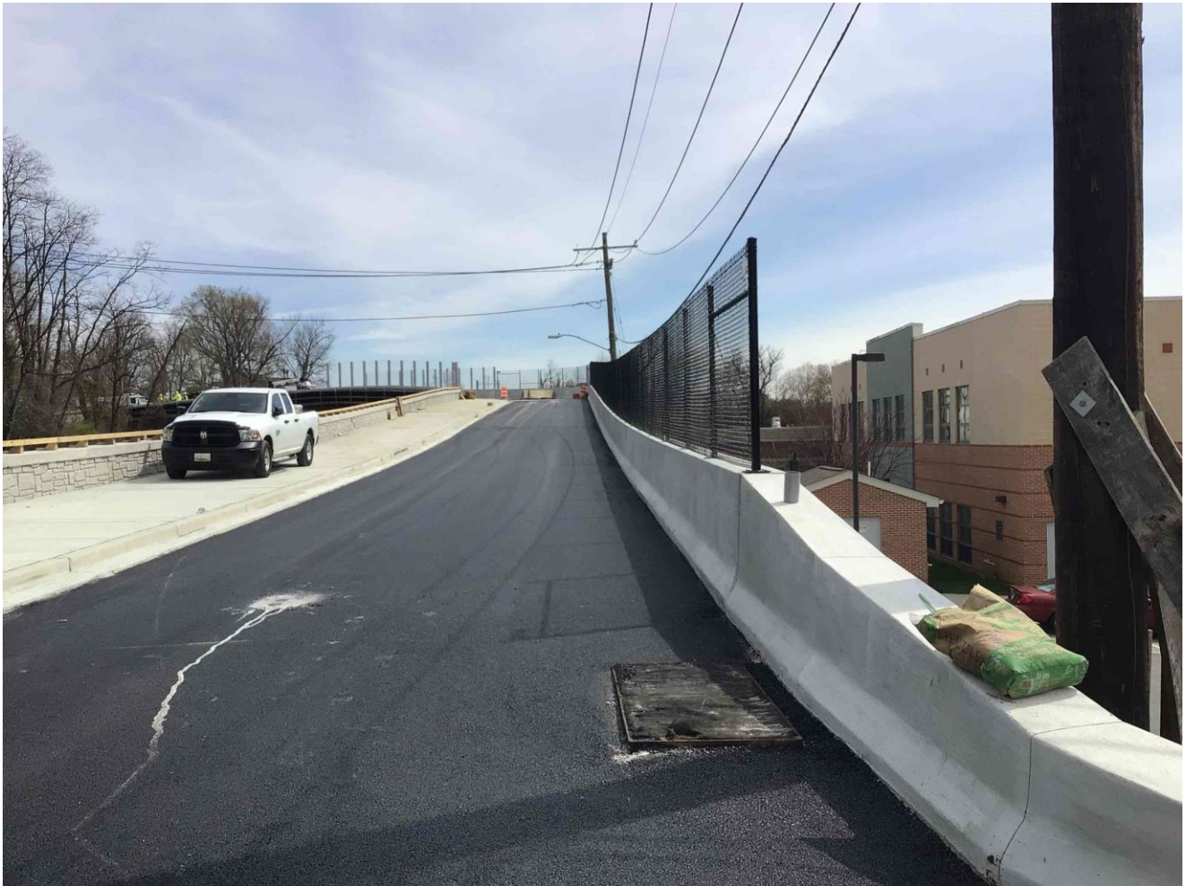
Segment 2: S18 Talbot Ave Bridge – Site view of the bridge approach pedestrian sidewalk and fencing work progress. (03.26.24)
