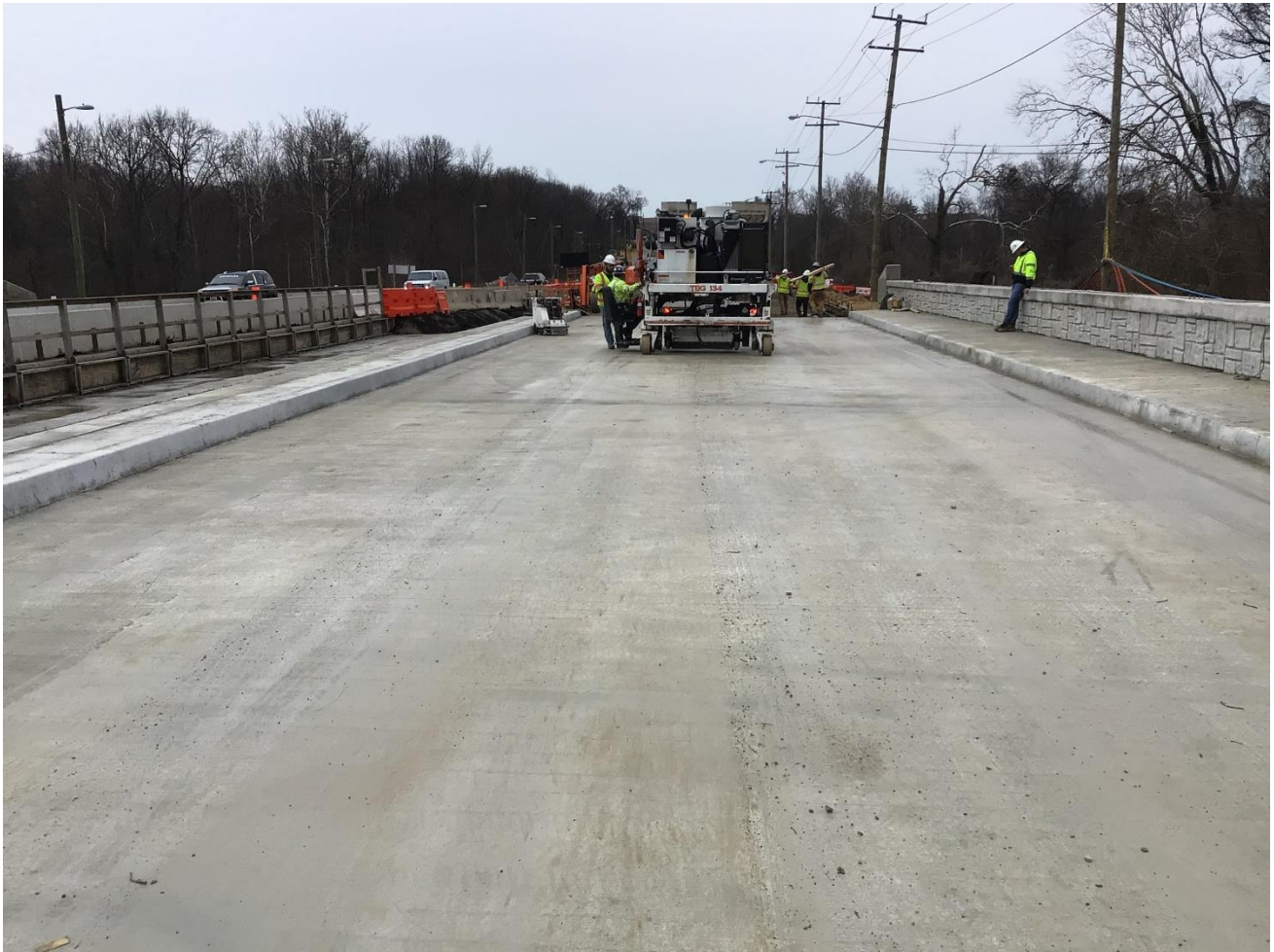
Segment 5: S27A/B NW Branch Bridge on University Blvd. – LRT bridge and traffic bridge site view of deck grooving work progress. (02.28.24)
