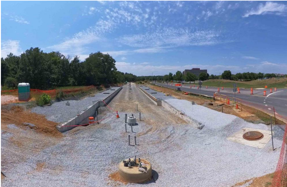
Segment 7 – Site view of Riverdale Park North UMD Station on River Road (07/13/23)
