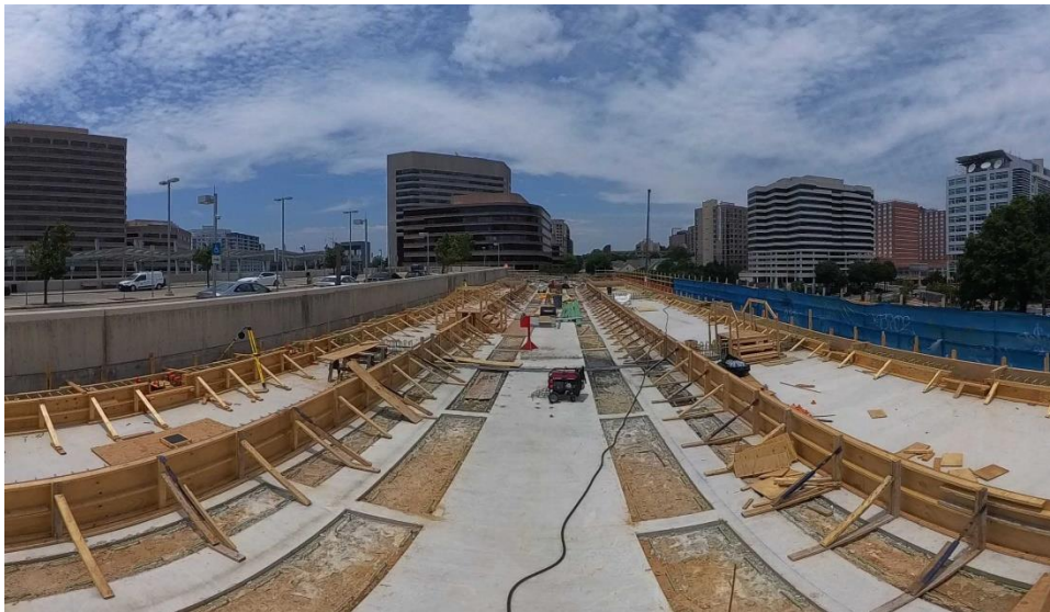
Segment 3 – Structure S20 LRT Bridge North & South Platform Formwork at Silver Spring Transit Center (07/13/23)
