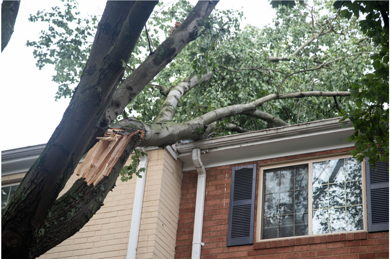
Thunderstorm damage, Maryland Adobe Stock
