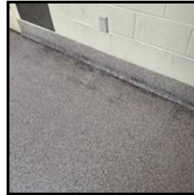
Uncleaned Floor and Wall
