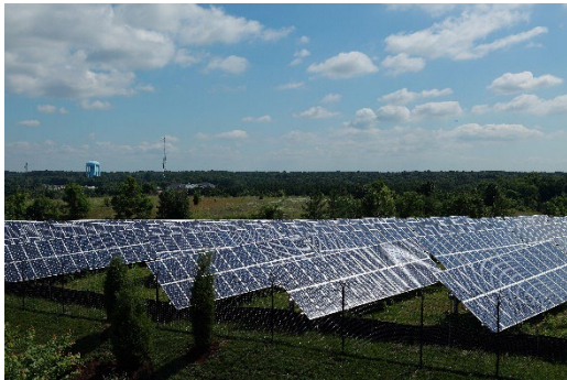
Solar Panels at MES HQ
