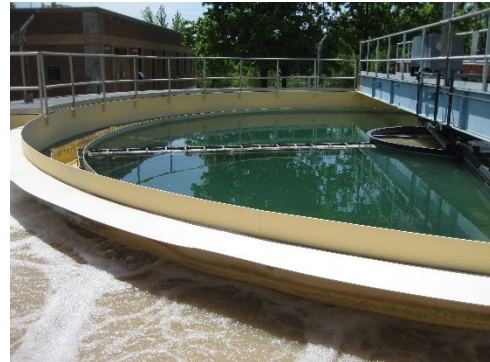
Dorsey Run WWTP
