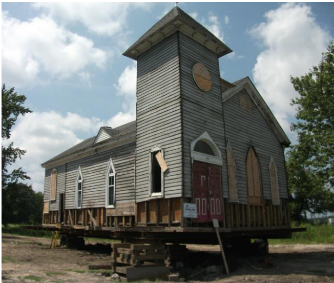
Above: Church during lifting and foundation repairs phase in the fall of 2012.
