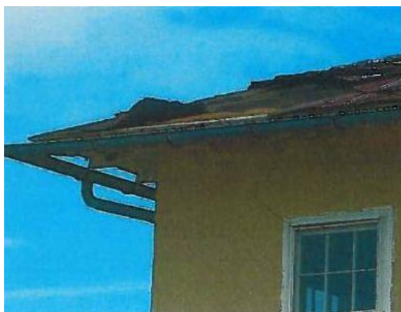
Hurricane Sandy-damaged roof in Crisfield.
