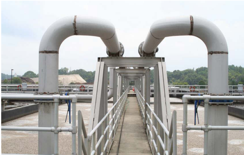
Sewage treatment along the Patuxent River.
