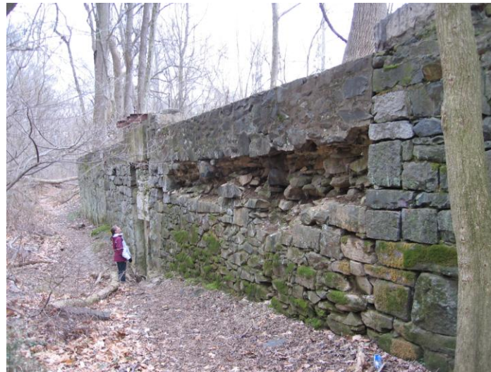
Staff examine industrial remnants associated with Savage Mill avoided by the path of the Little Patuxent Parallel Sewer.
