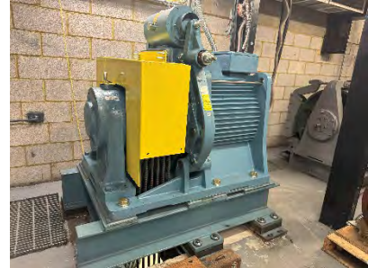
Figure 14 New Alternating Current Gearless Machine for WTC Elevator 7
