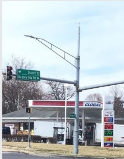
US 1 at MD 103 CCTV on Extension Pole
