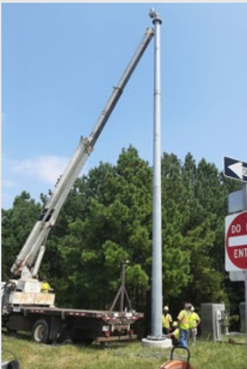
MD 175 at I-95 SB Ramp Stand Alone CCTV Pole
