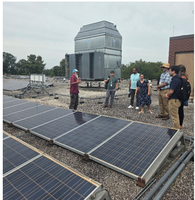
Staff of the Maryland Department of General Services and Maryland Energy Administration tour the solar roof of the Ellicott City MultiService Center
