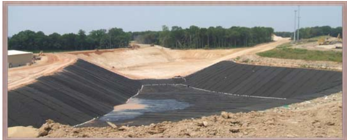
The construction of a new lined cell at Honeygo Rubble Landfill in White Marsh, Baltimore County
