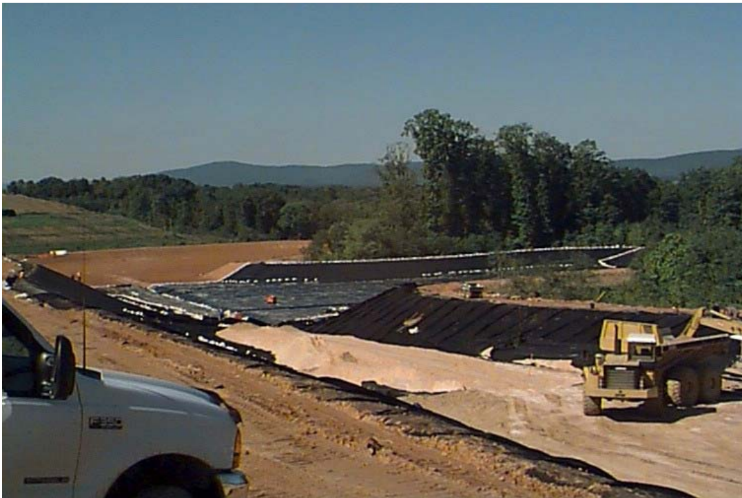
Picture 1. New lined landfill cell under construction in Western Maryland. Protective gravel drainage layer is being placed on low-permeability liner system.
