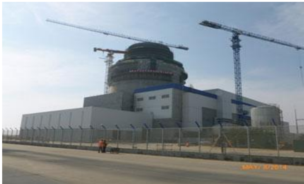
Figure 3-6 May 2014 Photo of the Construction of the Haiyang Nuclear Power Plant Units 1 and 2 in Shandong, China
