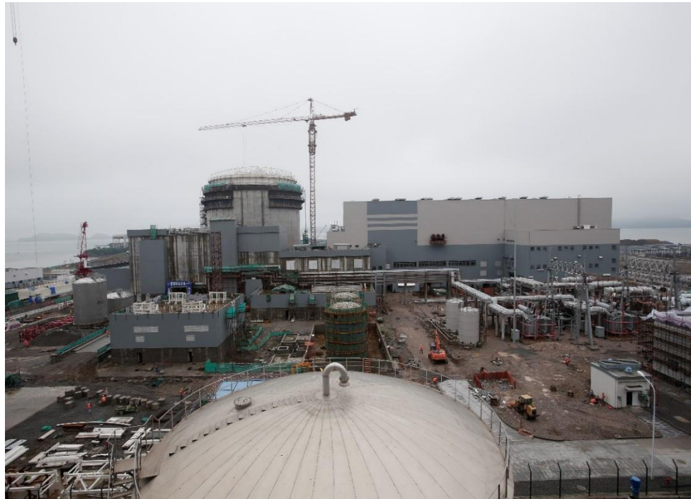
Figure 3-5 June 2014 Photo of the Construction of the Sanmen Nuclear Power Plant Units 1 and 2 in Zhejiang, China
