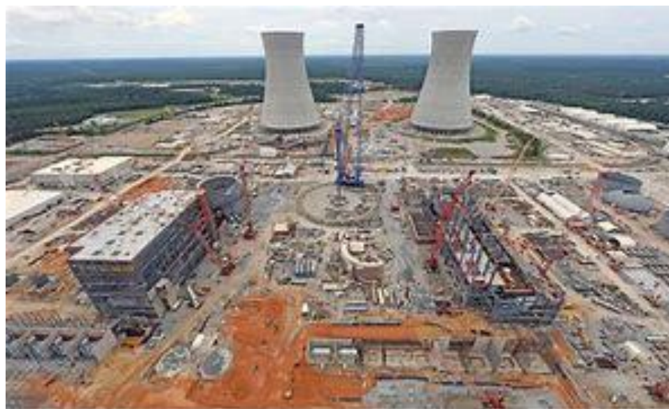
Figure 3-7 Photo of the Construction of the Vogtle Electric Generating Plant Units 3 and 4 in Waynesboro, Georgia
