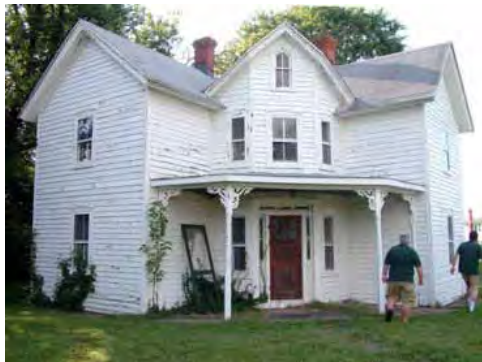
Once rehabilitated, the Lee House with its distinctive “W” façade will serve as the new home of the Tilghman Watermen’s Museum.
