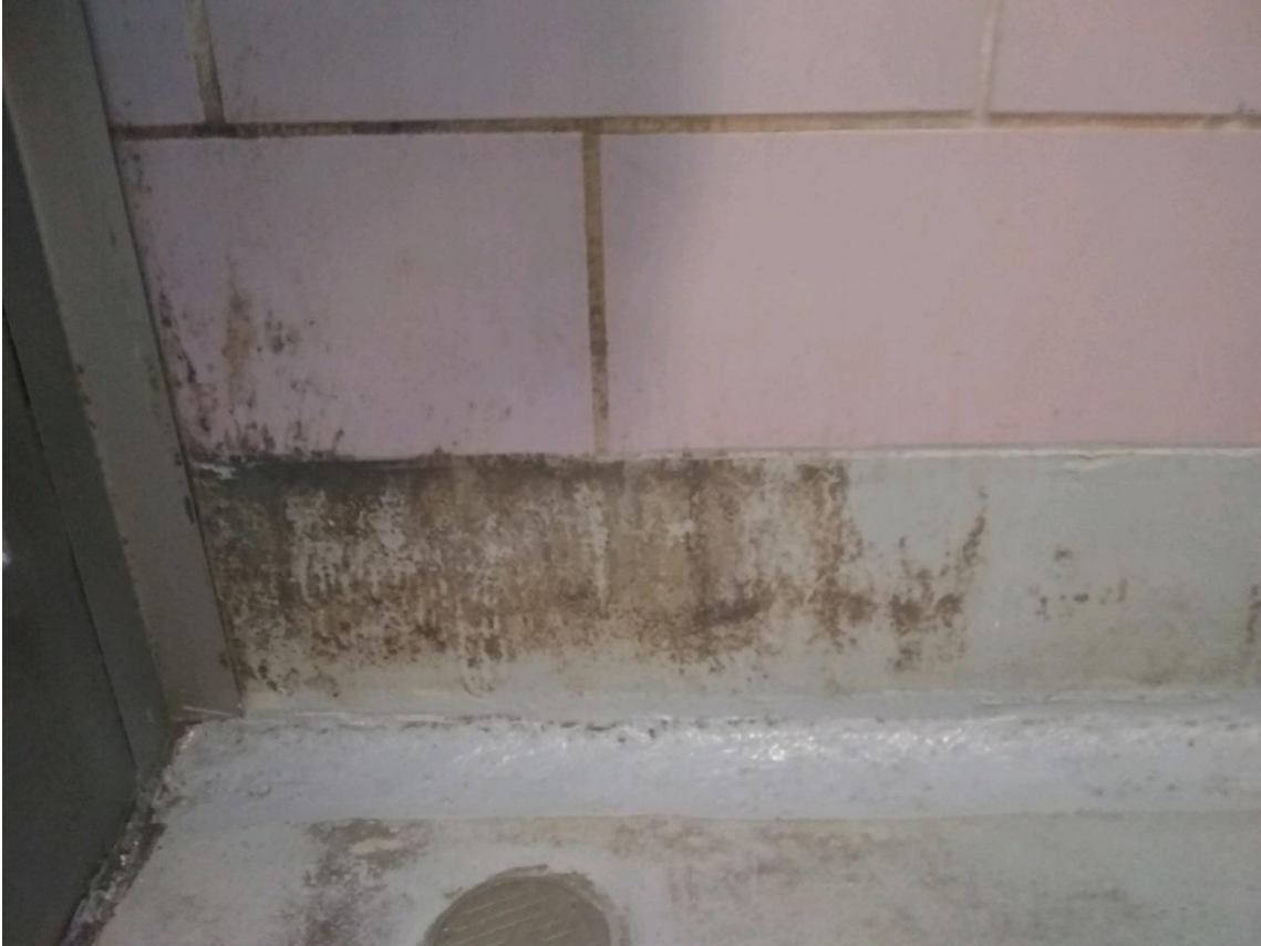
SHOWER WALL, FLOOR AND DRAIN FOR USE BY WAXTER RESIDENTS
